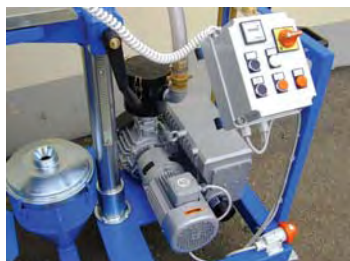
DETAIL OF ELECTRIC PANEL AND VACUUM PUMP
